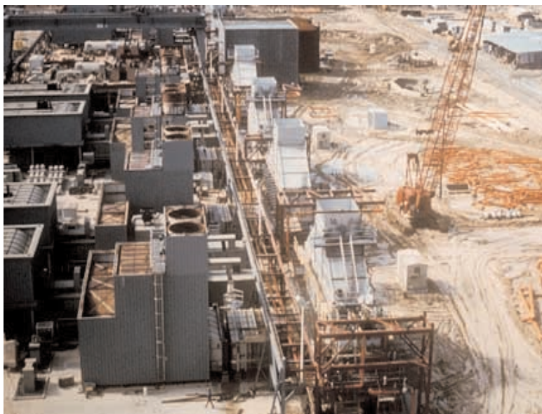
Figure 3. Two STAG 407B combined-cycle steam system installation
