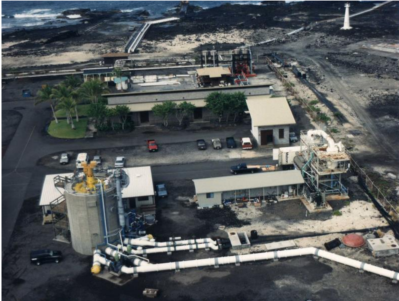
Pilot 250 kW installation at Kona Island (Hawaii)
